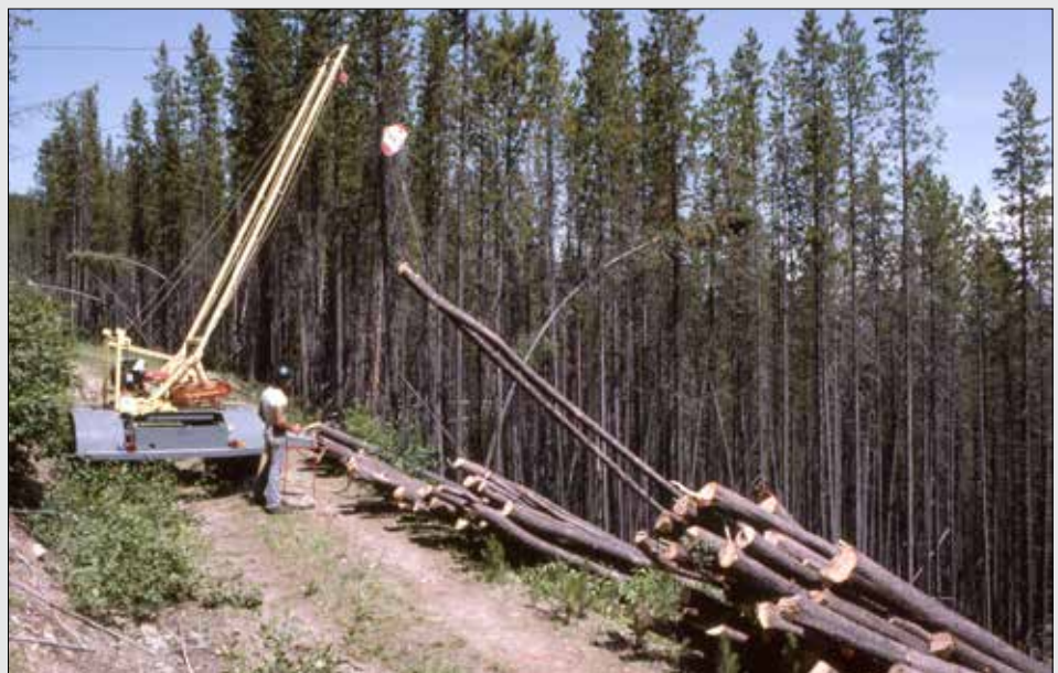
CLEARING SLASH Employees use a Bitterroot Mini Yarder, a low cost and mobile cable yarding system. The Bitterroot Mini Yarder is trailer mounted and pulled behind a pickup truck. (USDA)
